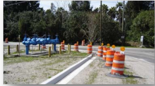
Gas Meters at John Rodes Blvd
