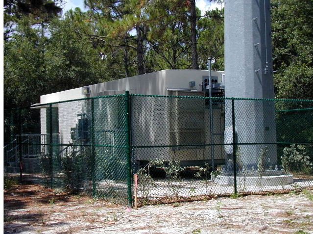
Figure 2: Example of 800MHz Wireless infrastructure Ground Equipment
