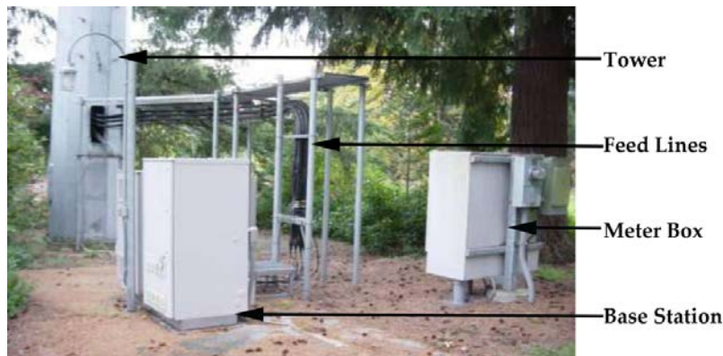
Figure 1: Example of 1900 MHz Wireless Infrastructure Ground Equipment
