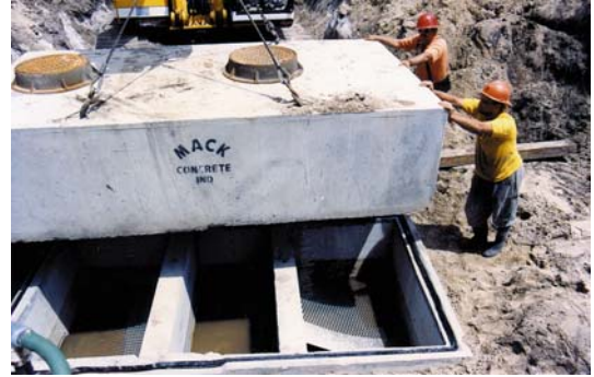
Installing a Baffle Box to reduce sediment and nutrients entering the Lagoon Photo by: Greg Jones, Brevard County NRMO
